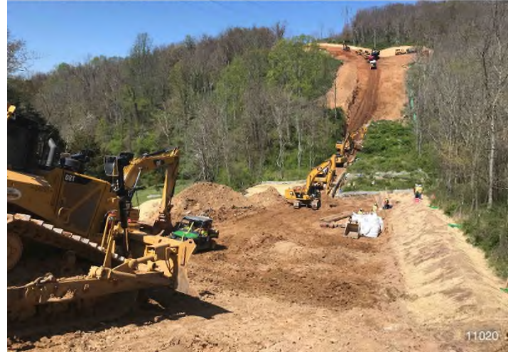
Figure 2: STA 11020+00 – Controls in place and functioning properly. BRG: 266°W (T) LAT: 37.323524 LON: -80.554245 ±16ft ALT: 2459ft
