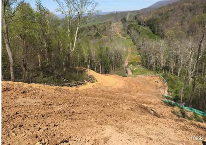
Figure 1: STA 10992+00 – Controls in place and functioning properly. BRG: 286°W (T) LAT: 37.325000 LON: -80.563064 ±16ft ALT: 2530ft
