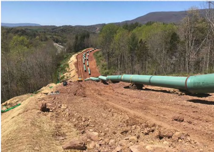
Figure 3: STA 11198+00 – Controls in place and functioning properly. BRG: 296°NW (T) LAT: 37.303724 LON: -80.505674 ±13714ft ALT: 2161ft
