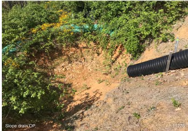
Figure 7: STA 11276+00 – Slope drain does not have outlet protection. BRG: 241°SW (T) LAT: 37.295868 LON: -80.487126 ±16ft ALT: 2281ft
