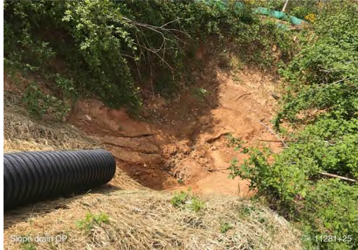
Figure 5: STA 11281+25 – Slope drain does not have outlet protection. BRG: 122°SE (T) LAT: 37.295792 LON: -80.485271 ±16ft ALT: 2273ft
