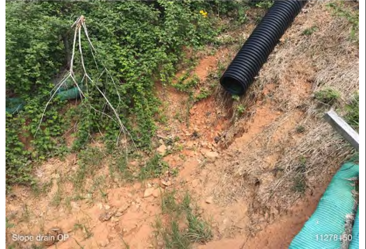
Figure 6: STA 11278+50 – Slope drain does not have outlet protection. BRG: 321°NW (T) LAT: 37.295762 LON: -80.486173 ±16ft ALT: 2241ft
