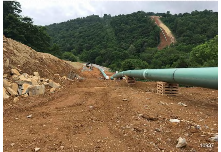
Figure 4: STA 10937+00 – Controls in place and functioning properly. BRG: 291°W (T) LAT: 37.330321 LON: -80.580914 ±16ft ALT: 2283ft
