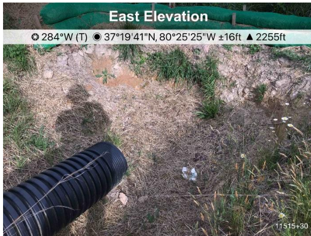
Figure 1: St 11515+30 sump lacks stone.
