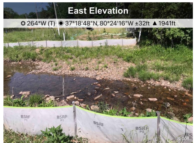
Figure 4: Designated crossing S-006, ECD's are in place.
