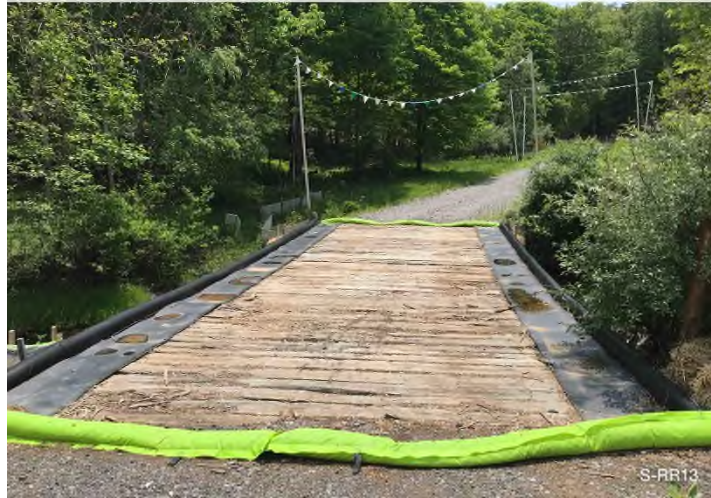
Figure 1: Stream S-RR13 – Controls in place and functioning properly around Craig Creek. BRG: 128°SE (T) LAT: 37.314629 LON: -80.402699 ±16ft ALT: 1878ft
