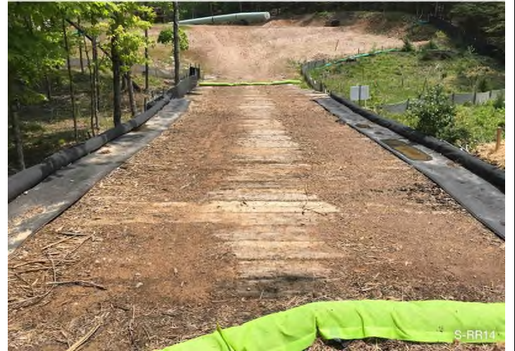
Figure 2: Stream S-RR14 – Controls in place and functioning properly around S-RR14 BRG: 110°E (T) LAT: 37.314042 LON: -80.402567 ±2805ft ALT: 1897ft
