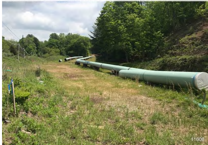
Figure 3: STA 11608+00 – Controls in place and functioning properly. BRG: 92°E (T) LAT: 37.313667 LON: -80.404540 ±32ft ALT: 1912ft
