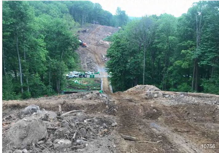
Figure 3: STA 10756+00 – Controls in place and functioning properly. BRG: 85°E (T) LAT: 37.344733 LON: -80.634306 ±16ft ALT: 2211ft
