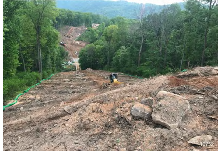
Figure 2: STA 10752+00 – Controls in place and functioning properly. BRG: 92°E (T) LAT: 37.344586 LON: -80.635579 ±16ft ALT: 2285ft
