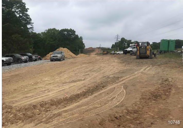
Figure 1: STA 10748+00 – Controls in place and functioning properly. BRG: 321°NW (T) LAT: 37.345255 LON: -80.636571 ±16ft ALT: 2301ft
