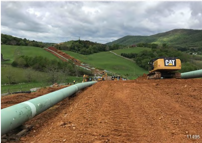
Figure 3: STA 11495+00 – Controls in place and functioning properly. BRG: 230°SW (T) LAT: 37.325289 LON: -80.429496 ±16ft ALT: 2288ft
