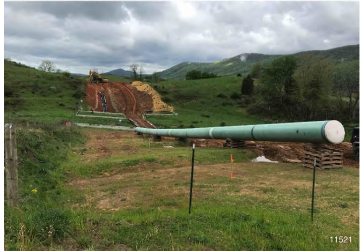
Figure 2: STA 11521+00 – Controls in place and functioning properly. BRG: 263°W (T) LAT: 37.328683 LON: -80.421833 ±16ft ALT: 2248ft
