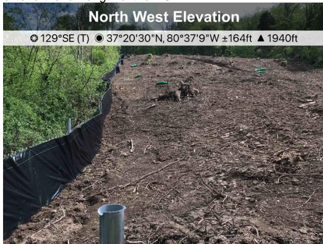
Figure 1: St10805+09 installation of waterbars uphill do not extend the full length of the ROW.
