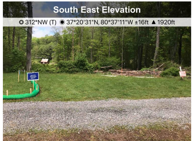
Figure 2: Designated crossing S-Z14, ECD's are in place.
