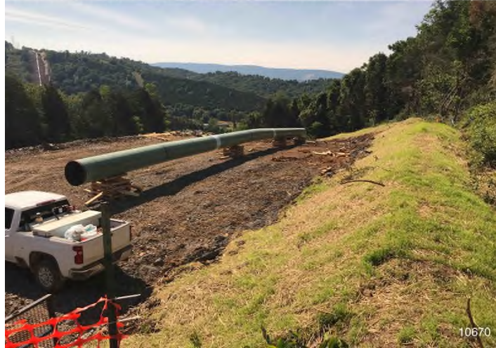
Figure 1: STA 10670+00 – Controls in place and functioning properly. BRG: 142°SE (T) LAT: 37.351245 LON: -80.660704 ±16ft ALT: 2256ft
