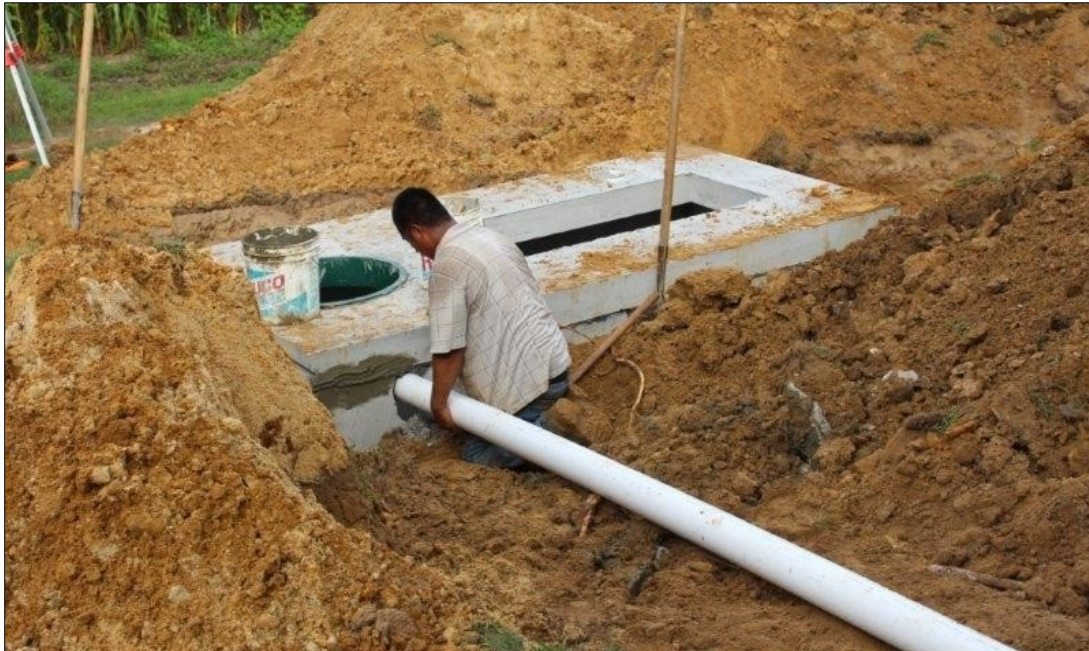
Figure 2: Connecting home sewer line to new alternative onsite sewage system, Matthews County, Virginia (Courtesy of VDH)
